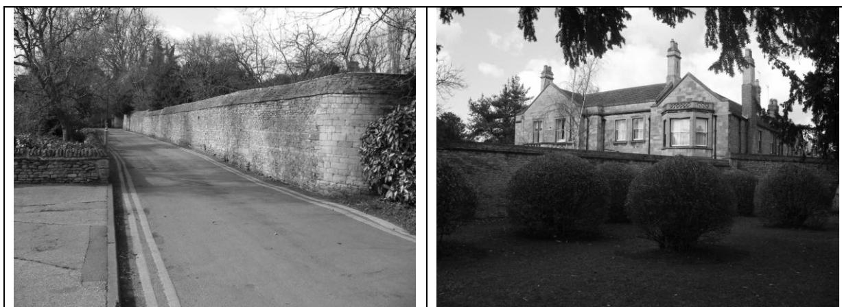
The Precinct boundary wall along Gravel Walk looking west (left), and along the east side with the Vineyard behind it (right, looking north-west).
