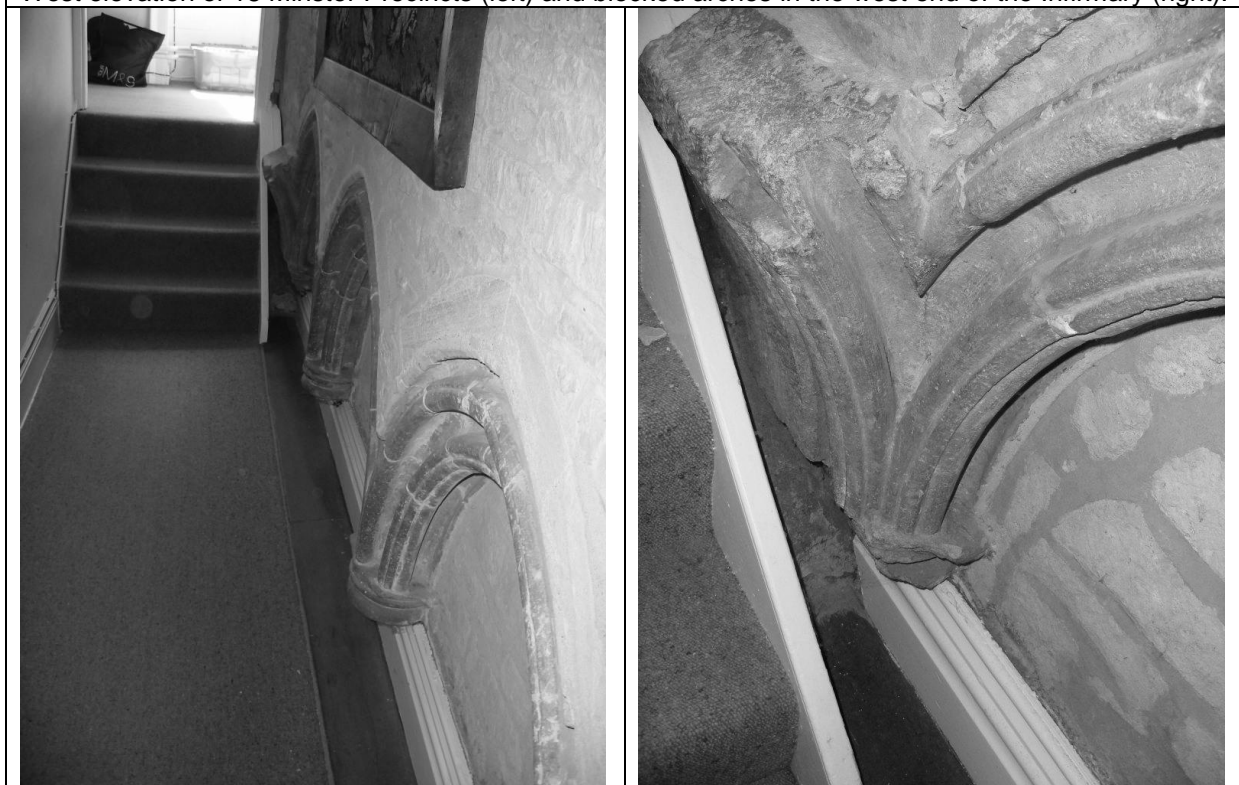
The arches at the west end of the Infirmary Hall's south aisle (left), with a detail of the return arch springing (right).
